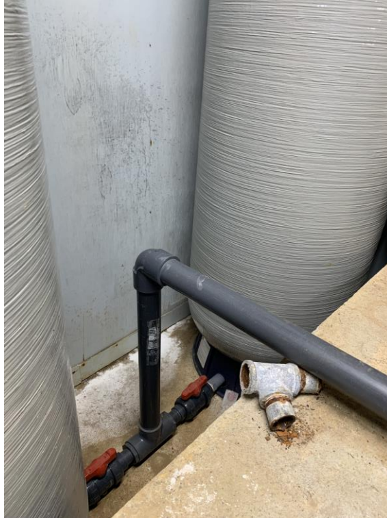
Figure A.21: Connection to East (Newer) Pressure Tanks and Isolation Ball Valves
