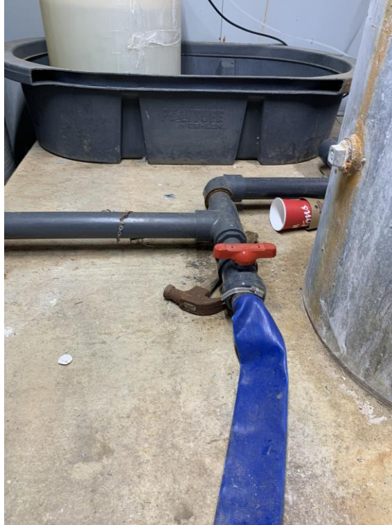
Figure A.19: Flexible Hose Connection to Pressure Tank PVC Header Piping
