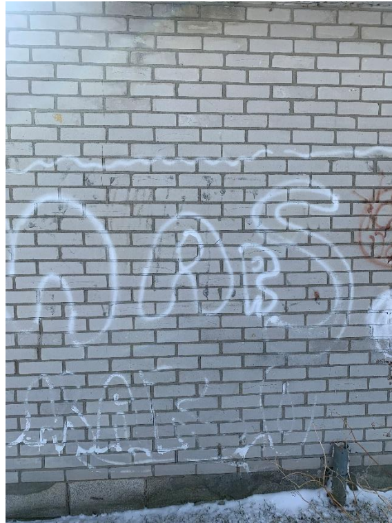
Figure A.3: WTP Exterior Wall Showing Ageing of Bricks and Graffiti
