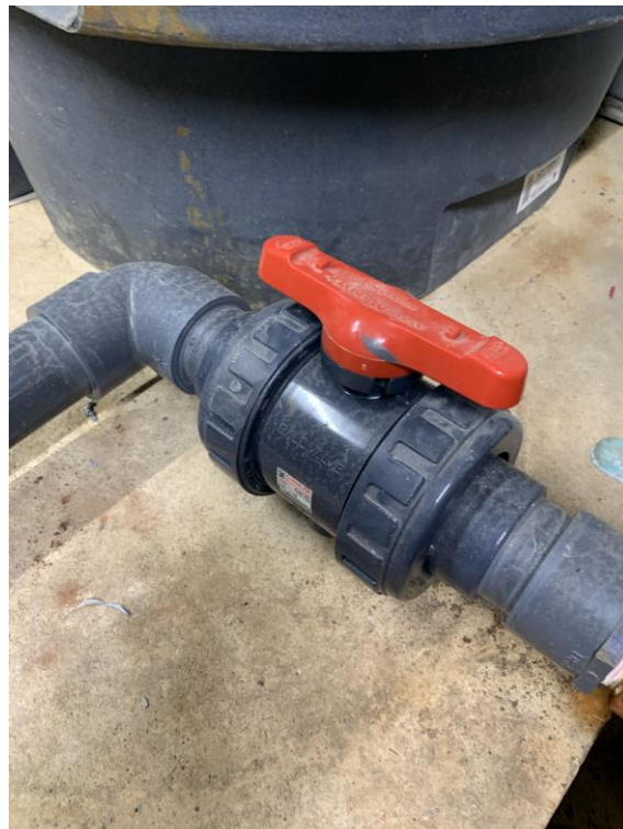
Figure A.18: Isolation Ball Valve on PVC Header to the Two East (Newer) Pressure Tanks
