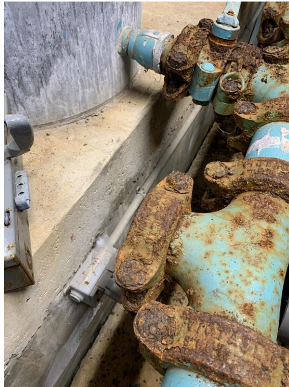
Figure A.17: Header Piping to the Two West (Older) Pressure Tanks. The Piping Shows Significant Corrosion
