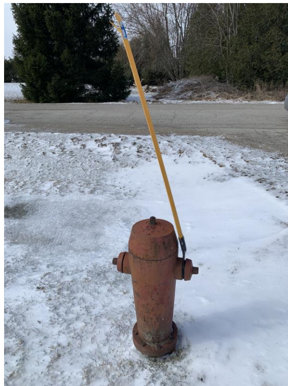
Figure A.26: Hydrant on Grand Crescent in Front of the Water Treatment Plant
