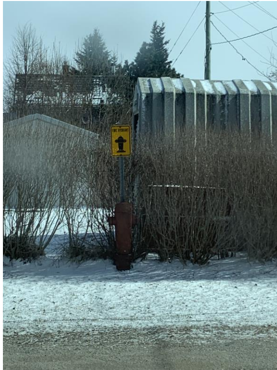
Figure A.27: Hydrant on Grand Crescent Near Intersection with Orangeville-Fergus Road
