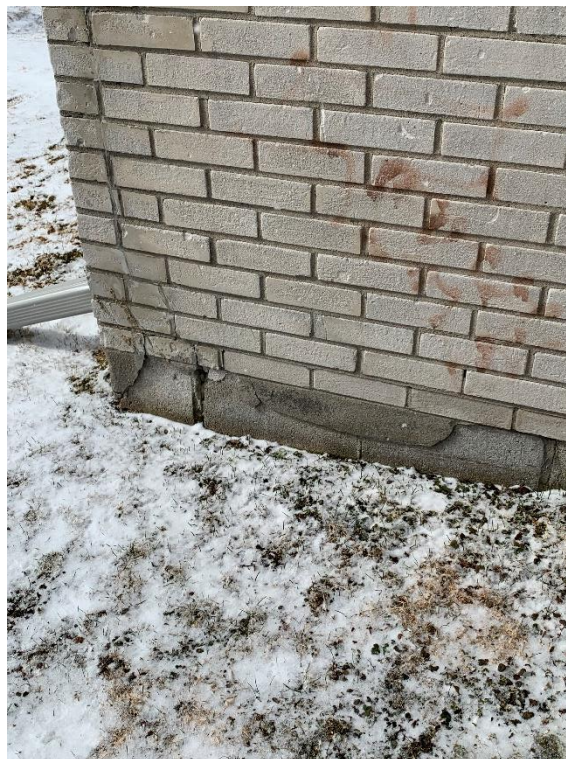
Figure A.4: WTP Exterior Wall Showing Minor Cracks in Foundation and Damage to Bricks
