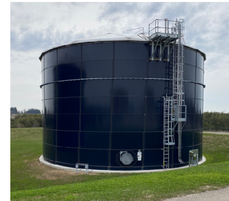
Example of Storage (Standpipe)
